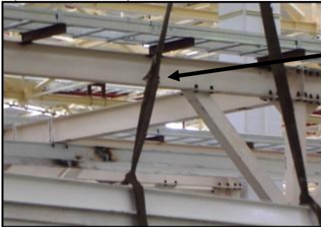
Rope sling damage
